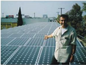
GJ Electric Solar's Joe Gamiel points at the solar system his company installed at Valley Car Wash.
