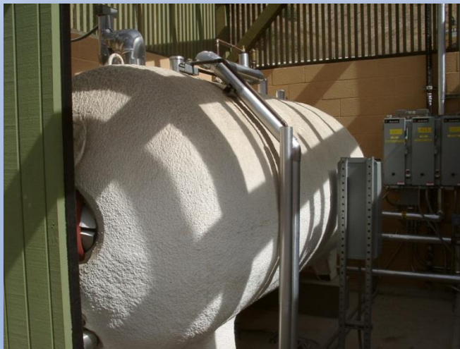
Hot Water Storage Tank
